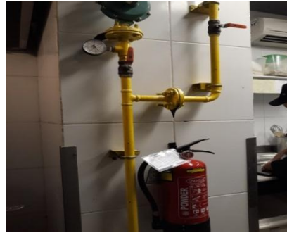
Pipa Gas & APAR
