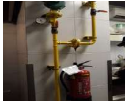
Pipa Gas & APAR
